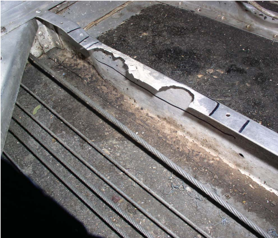
Severely compromised floor structure. This area should be inspected at every annual.
