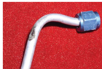
Corroded fuel line.
