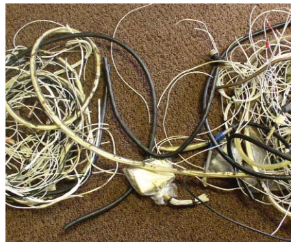
All this unused old wiring was hiding behind the side panels.
