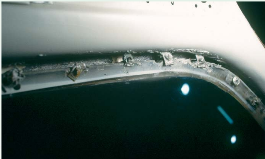
A disastrous window installation with many holes on or 1/2 inch off the edge of the Plexiglas.
