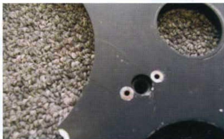
An 8-32 nutplate installed in an oversized hole.
