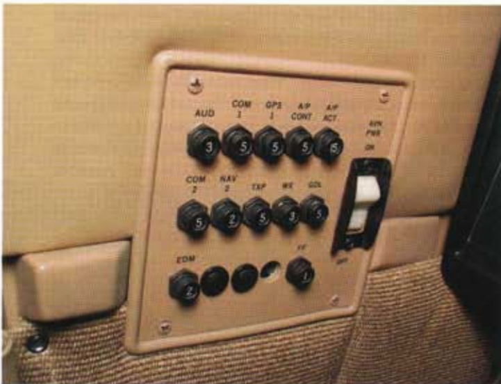
Renovated side panel circuit breaker panel.
