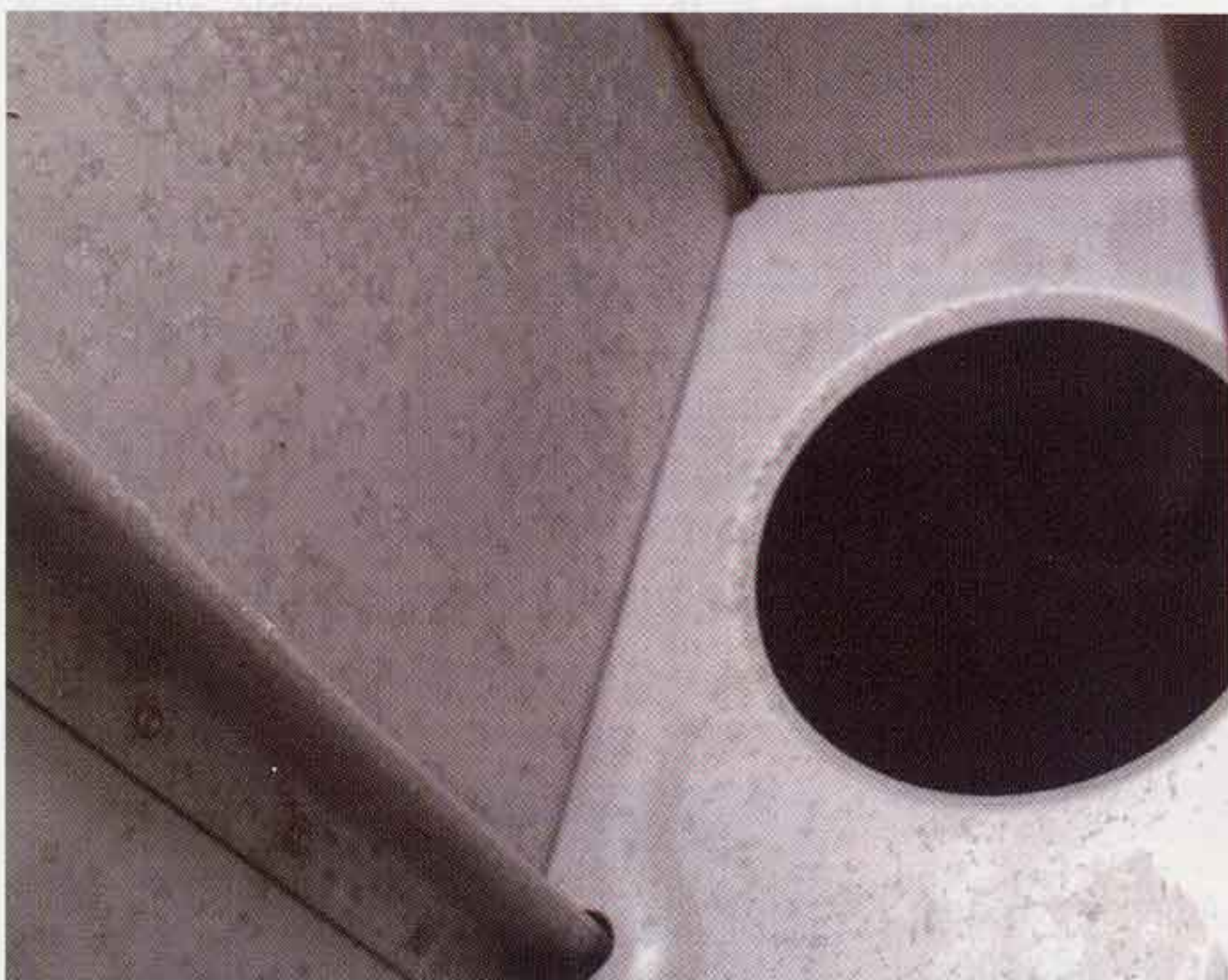
Figure 1—Surface corrosion caused by moisture and airborne contaminants attacking an unpainted bare aluminum surface.
