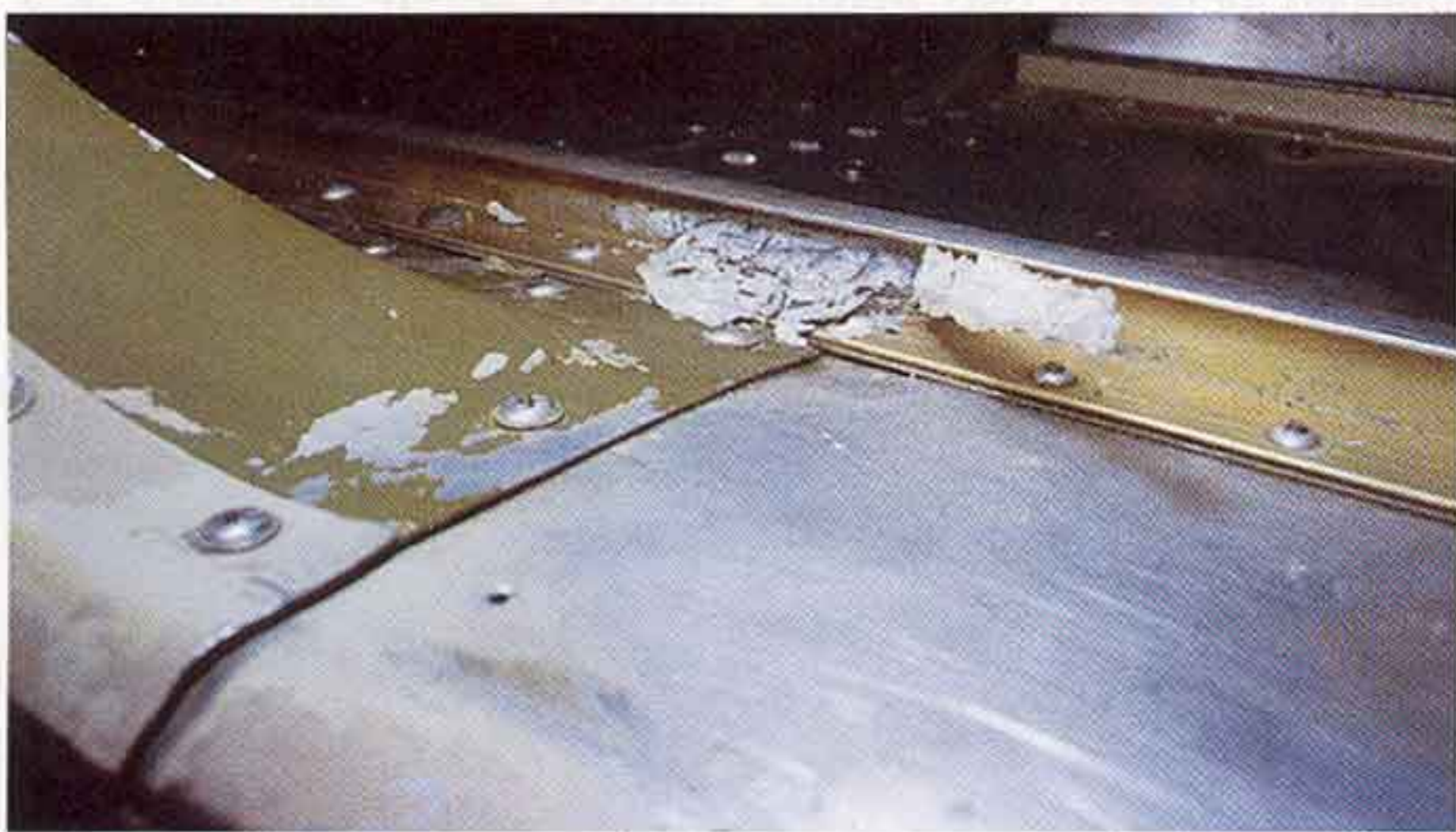
Figure 5—Inner granular corrosion
