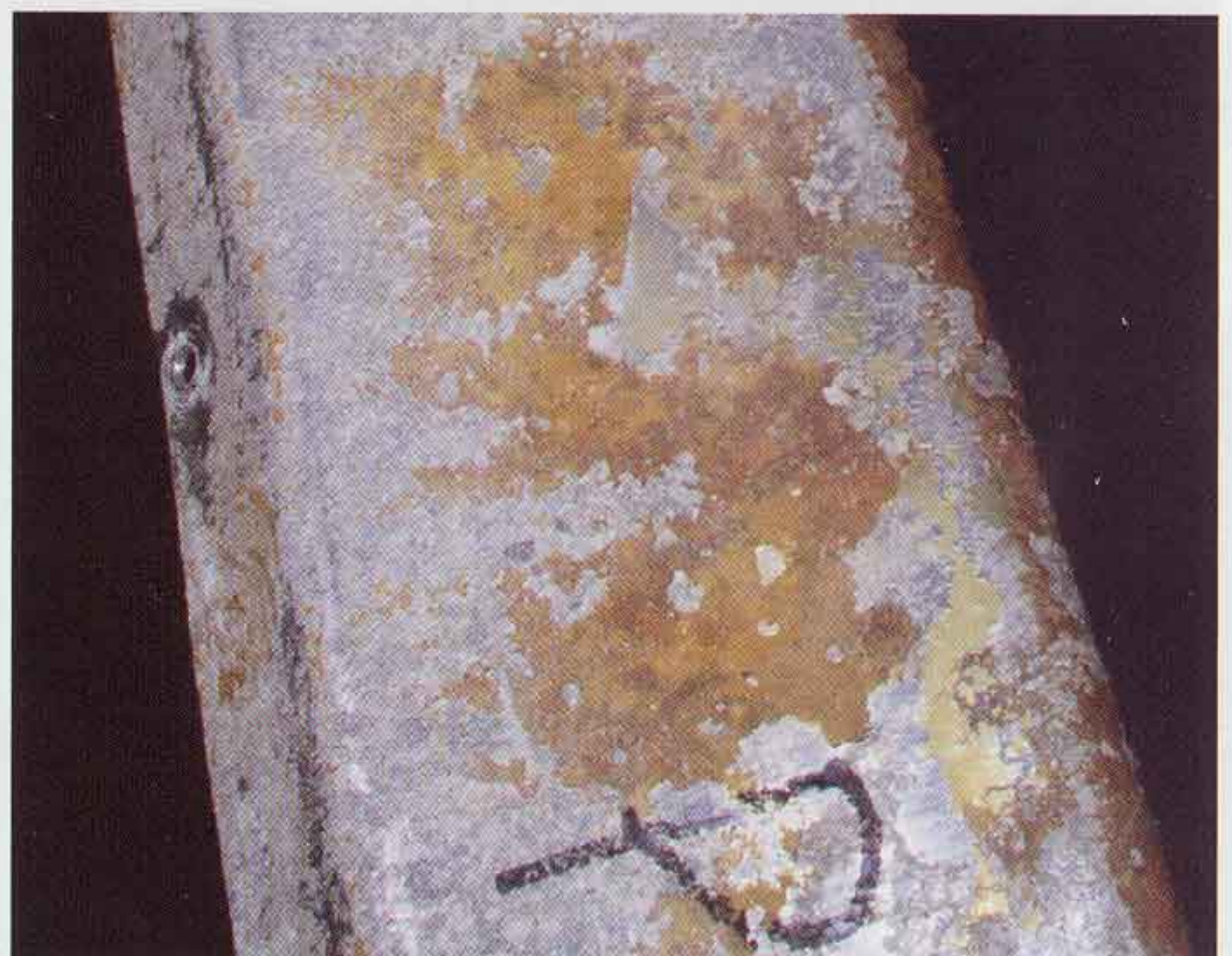
Figure 2—Surface corrosion exacerbated by a hydroscopic glue being applied to a bare aluminum surface.
