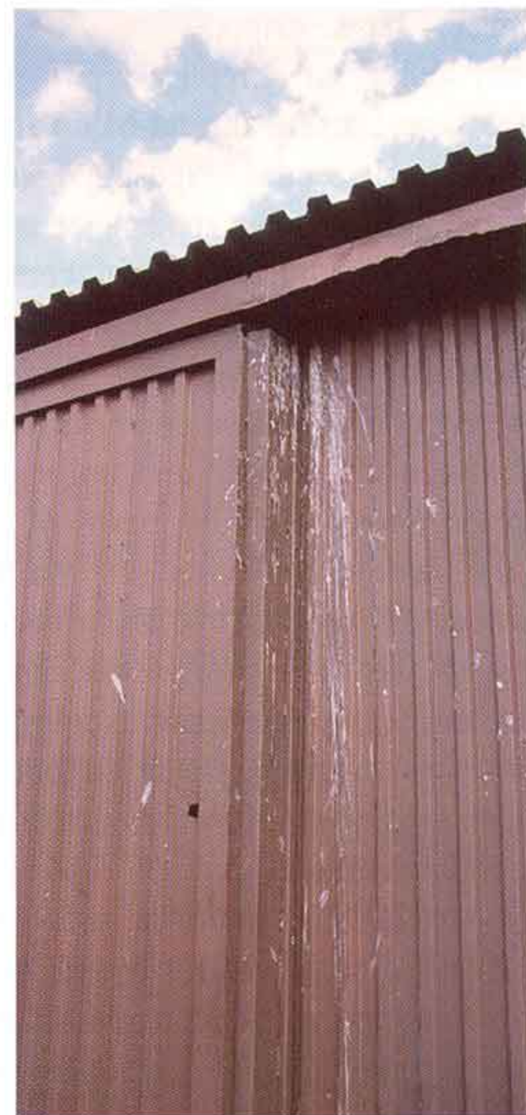
Evidence of birds getting into hangar. Animal urine is very corrosive.
