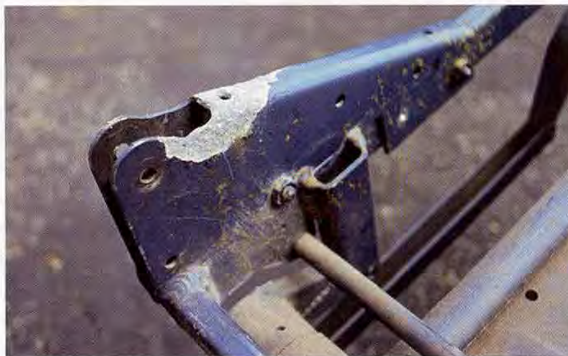
After-market flame treatments for upholstery materials are likely to cause corrosion, as in the photo above.
