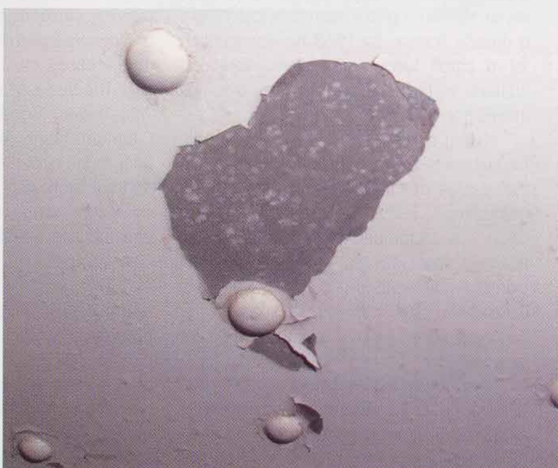
Figure 4—Surface corrosion that started as filiform corrosion, then the paint split open and surface corrosion spread at will on the skin's surface.
