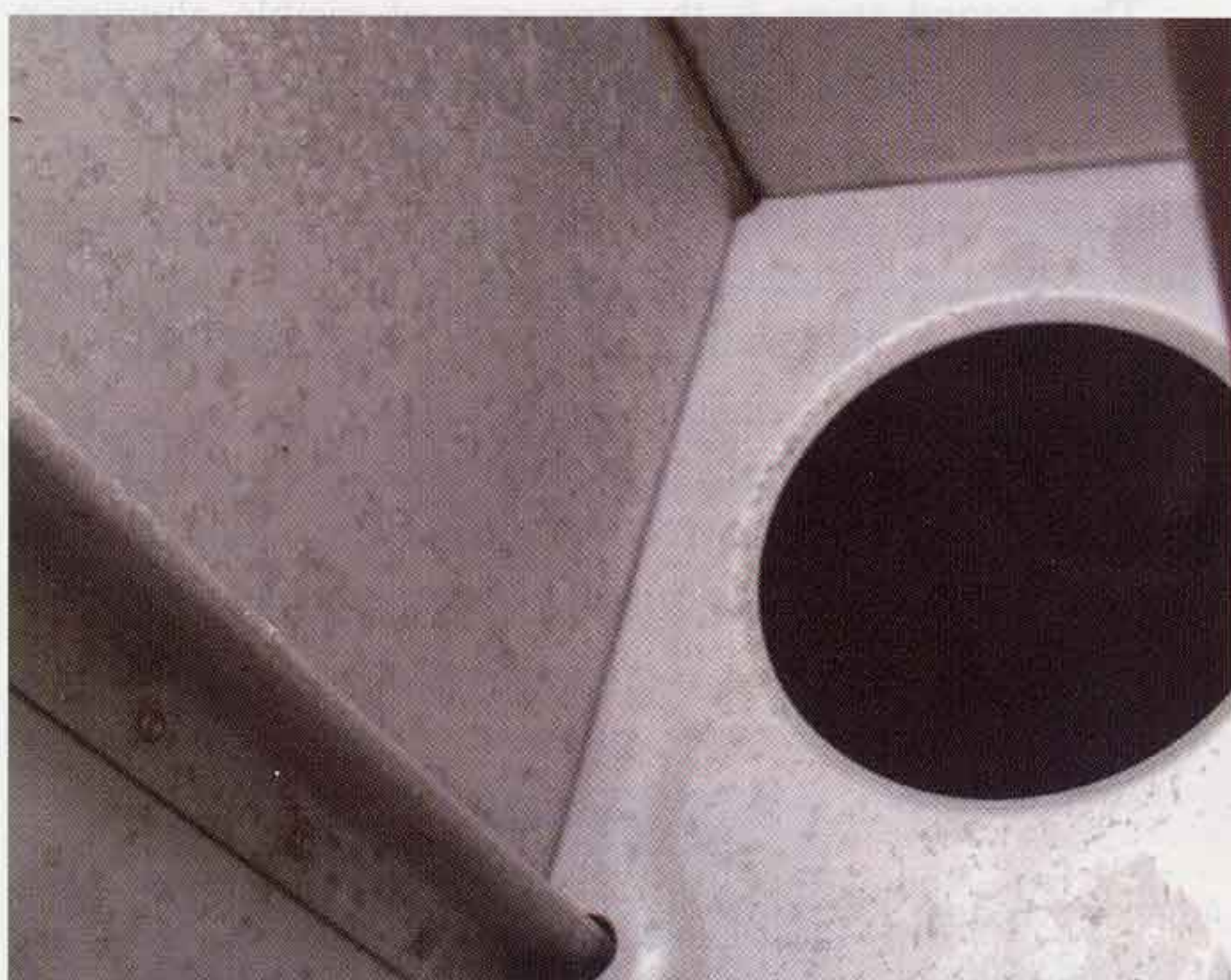
Figure 1—Surface corrosion caused by moisture and airborne contaminants attacking an unpainted bare aluminum surface.
