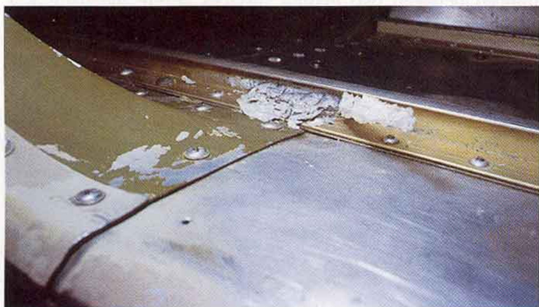
Figure 5—Inner granular corrosion
