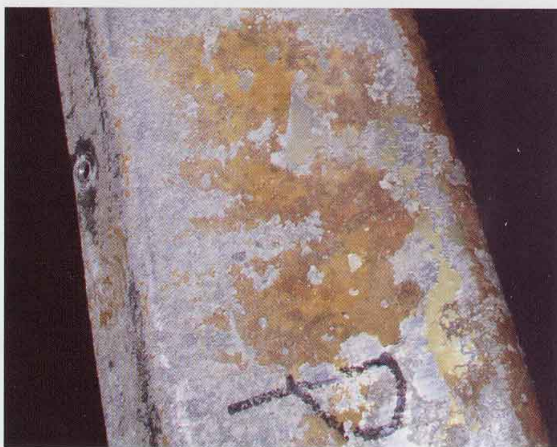
Figure 2—Surface corrosion exacerbated by a hydroscopic glue being applied to a bare aluminum surface.
