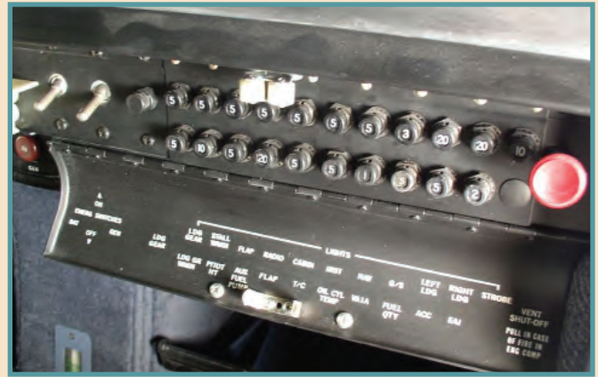
All the main ship's buss circuit breakers are laid out in one accessible location.
