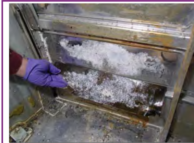
I just had to show another picture of the lead-vinyl/corrosion problem.
