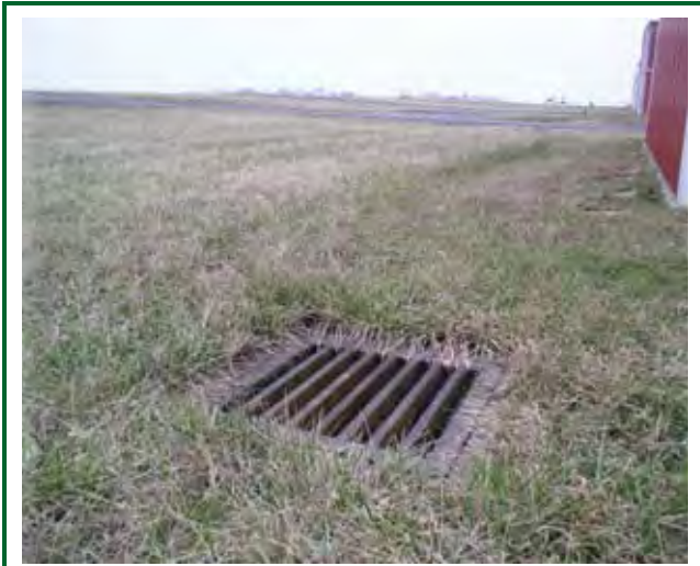
A storm drain located between high ground and T-hangar. Check it out before you rent.
