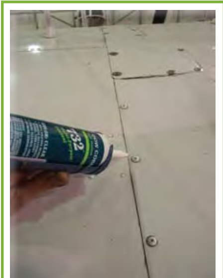
Dow Corning non-corrosive 732 silicon caulk seals the wing and fuselage seams.
