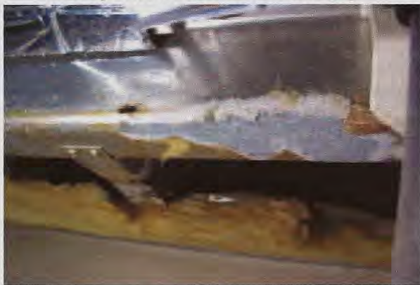
Corrosion on the surface of the aft spar carry-thru where the contaminated headliner touched it
