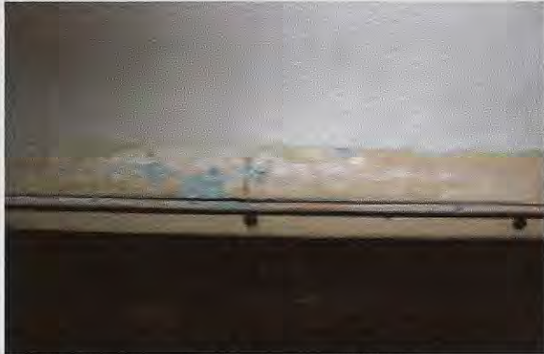
Severely corroded headliner retainer strip
