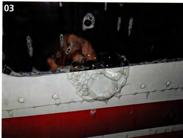
Leaking windows is another non-upholstery issue common to aging Pipers.
