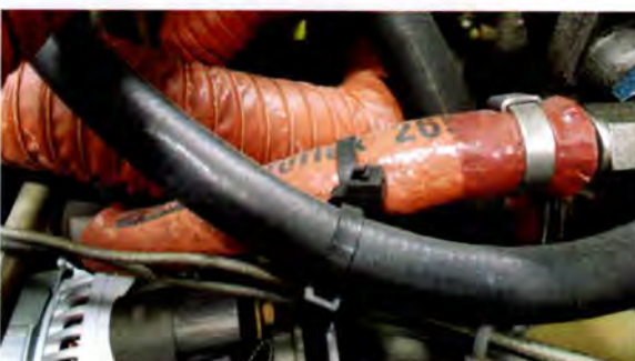
Incorrect use of plastic tie wraps, intended to prevent two hoses from rubbing against one another.
