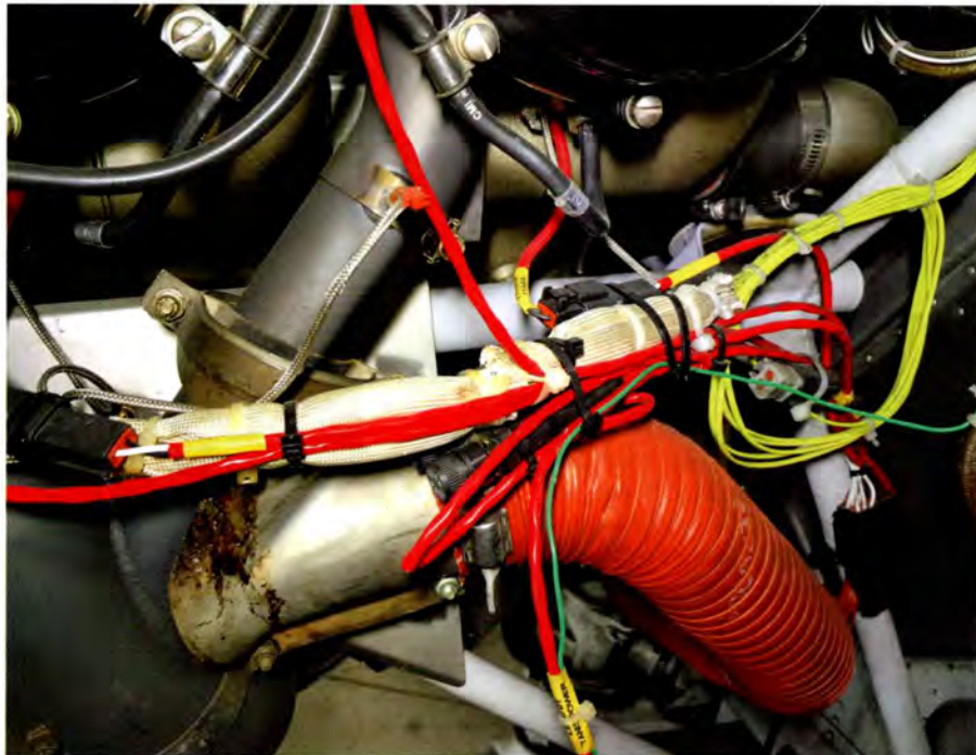
A typical collection of instrument wiring. These wires go to temperature gauges for measuring cylinder head, exhaust, oil and carburetor temperatures.
