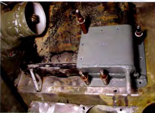
A stainless steel battery box with a welded corner repair, ready to be sealed with epoxy seal material secured with rivets.
