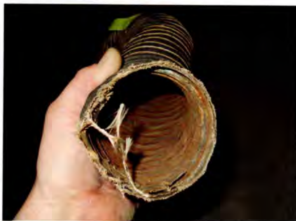
Deteriorated neoprene-impregnated fiberglass duct hose; replace this stuff with better quality orange silicone SCAT duct hose.
