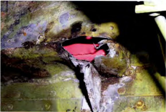
Severe battery acid damage in the lower corner of an aluminum battery box.
