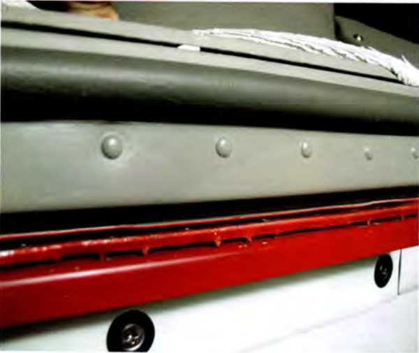
The white headliner material at the top of the photo is being pulled out of the retaining rail, inch by inch.
