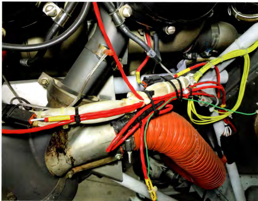
A typical collection of instrument wiring. These wires go to temperature gauges for measuring cylinder head, exhaust, oil and carburetor temperatures.
