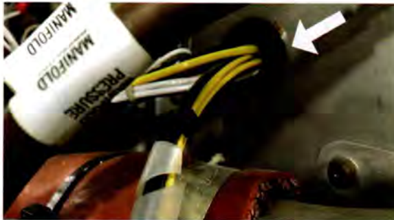
A simple rubber grommet is not the correct method for running a wire through a bulkhead.
