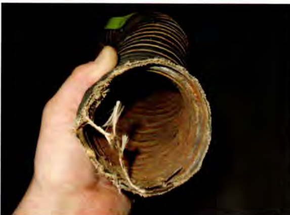
Deteriorated neoprene-impregnated fiberglass duct hose; replace this stuff with better quality orange silicone SCAT duct hose.
