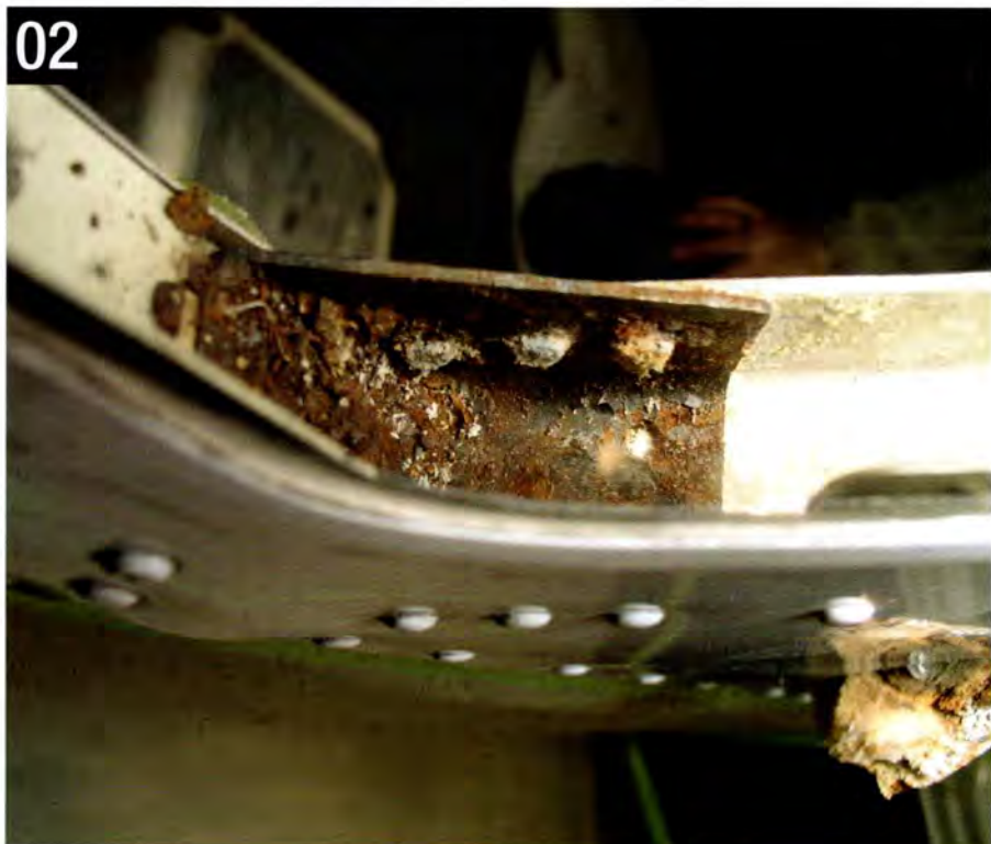
Obvious rust on a steel reinforcement bracket. An inadequate pre-purchase inspection may miss something like this.
