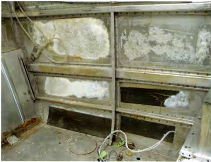
Corrosion caused by galvanic action under glued-in-place lead vinyl skin damping panels.
