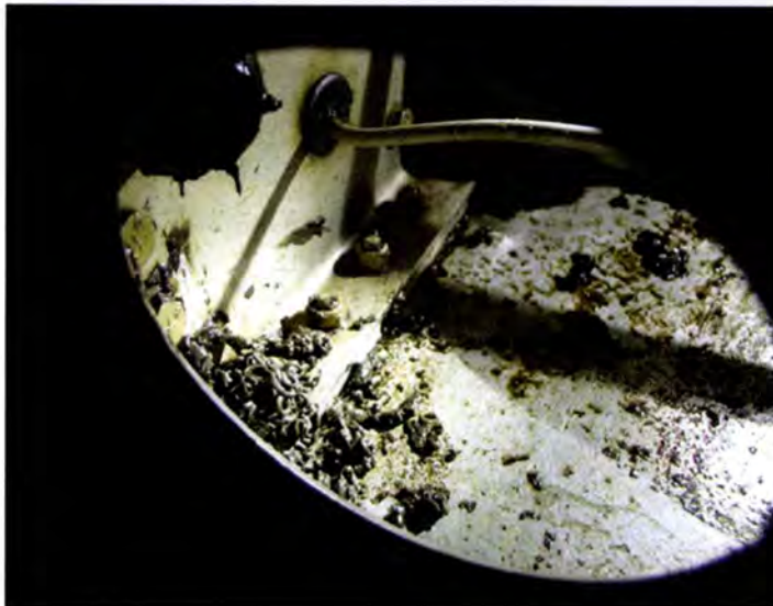
Extensive corrosion on belly skin caused by dirt.
