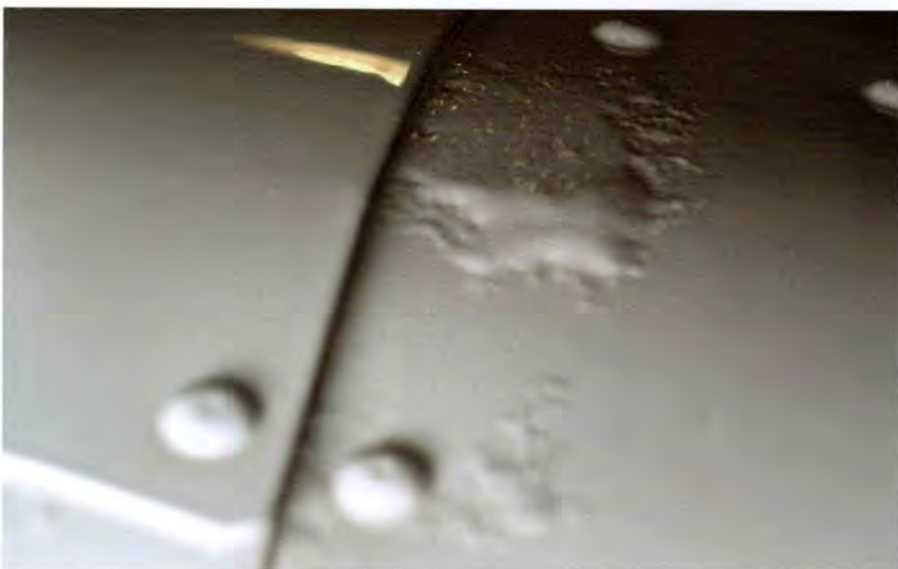
Filiform corrosion creeping out under the paint of an improperly cleaned lap joint. The joint should have been more carefully cleaned prior to applying primer and finish paint.
